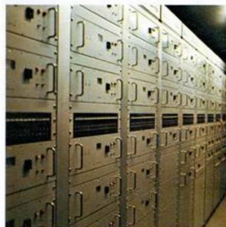
Neatly-stacked rows of 160 unit power amplifiers.
