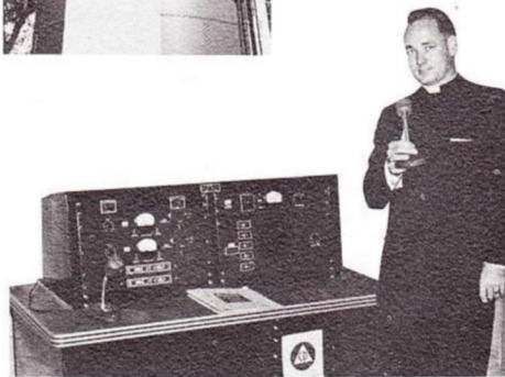
Controls for the Giant Voice Warning System may be centrally located in a CITY HALL, POLICE DEPARTMENT, or COMMUNITY CENTER. Shown above is a tornado and flood warning system used in Crockett, Texas.
