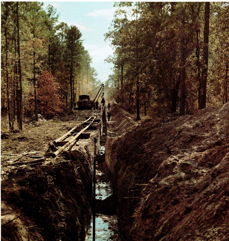
Texas Eastman built a 275-mile pipeline between its plant in Longview and gas storage facilities near Houston. Eight pipelines now connect Texas Eastman with sources of the petroleum gases it uses to make polyolefin plastics and industrial chemicals.
