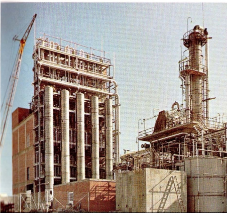
This plant at Tennessee Eastman will produce terephthalic acid for use in making Tenite polyester plastic, Kodel fiber, and Estar film base.
